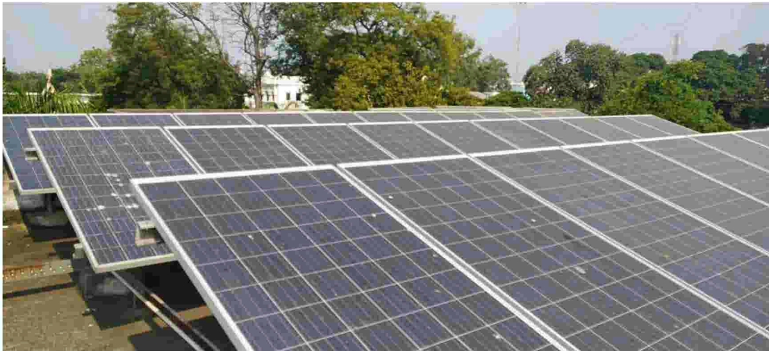
Fig: Grid connected Solar PV Plant at Computer Lab
